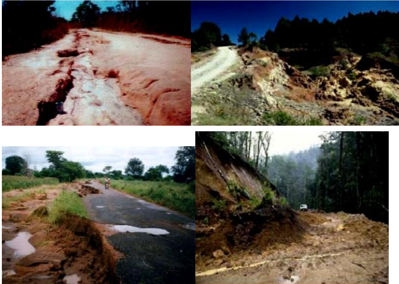
Figure 10: Slope failure in Highway due to improper drainage system
