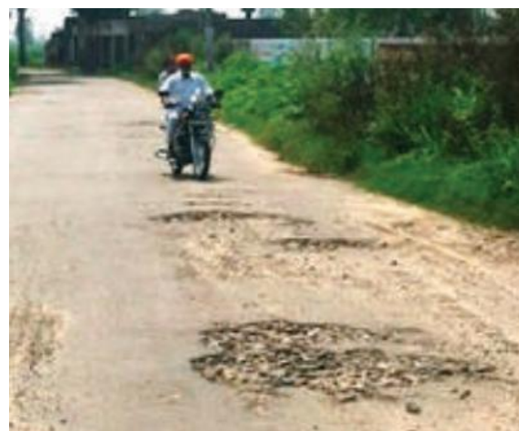
Figur 2.3: Potholes on road
